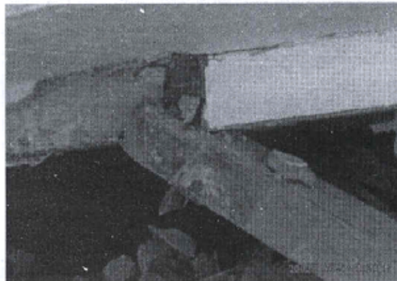
Fig. 18: Weak connection between beam and column
