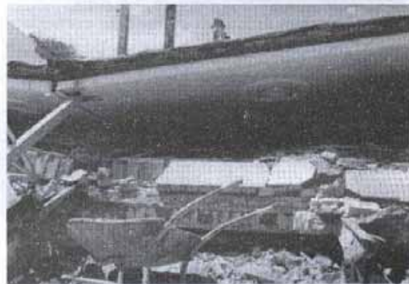
Fig. 14: Collapsed simple steel frame building
