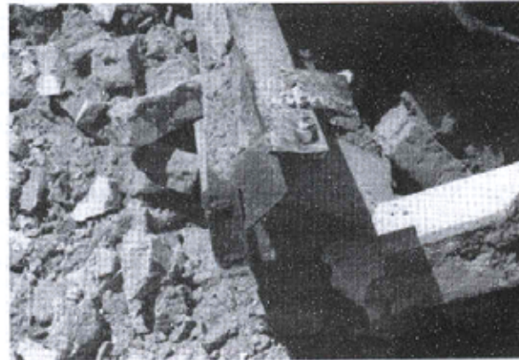
Fig. 12: Failed jack arch roof
