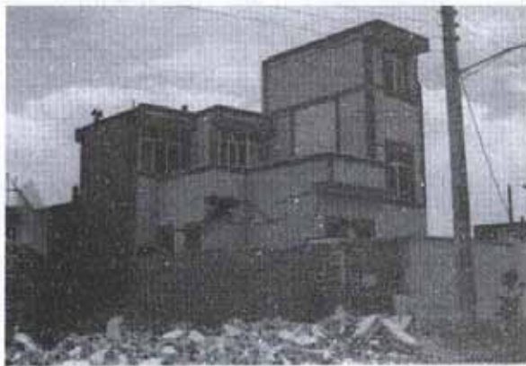
Fig. 13: 3-story steel frame building damaged due to high torsional forces
