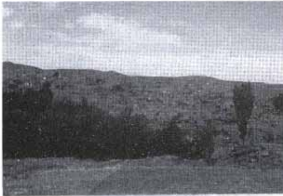
Fig. 7: Complete failure of adobe buildings in Abdarreh
