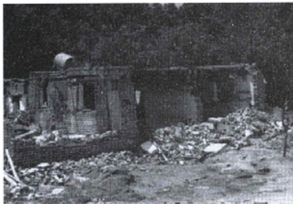
Fig. 11: Damaged brick masonry building
