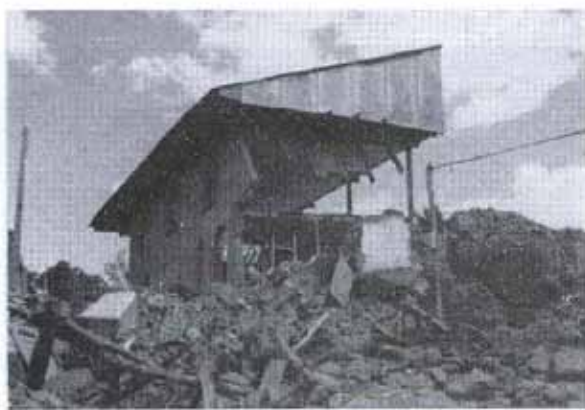
Fig. 15: Collapsed simple steel frame building
